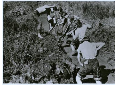
Fig. 4 Students working on drainage ditch for the Studies Building, Lake Eden Campus, ca. 1940-41. Courtesy of the Western Regional Archives, State Archives of North Carolina.
